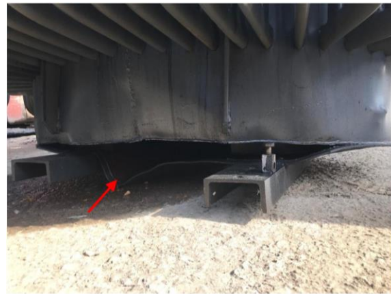
Figure-2: Transformer Bottom Plate Rupture
