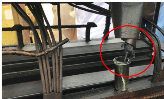
Figure-3: HT Side Terminal Connection
