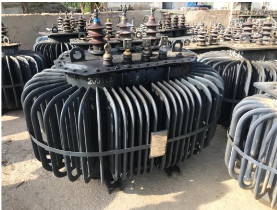
Figure-1: 200kVA Transformer
